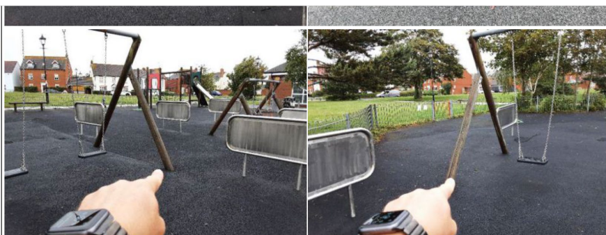
Finding: Two of the posts have rotted and the remaining timber is showing signs of rot Action: Replace all rotted timber
